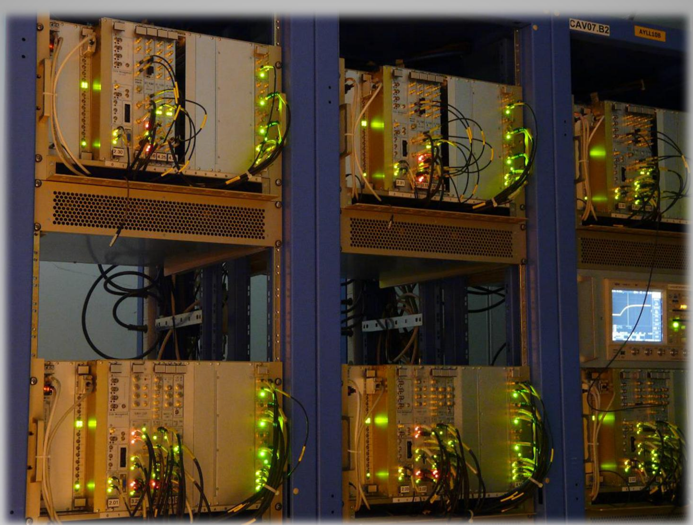
One Rack contains 1 complete cavity controller
