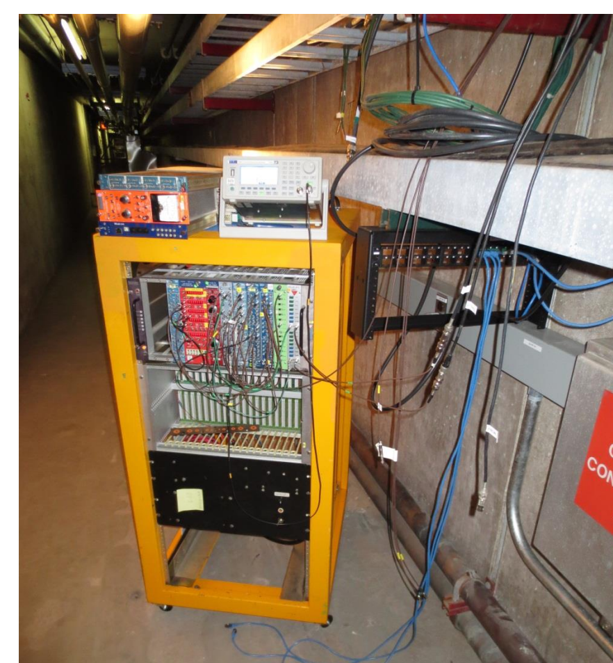
Network panel in Beam Enclosure
