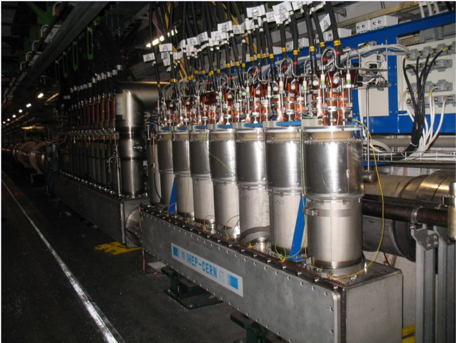
DFB in the tunnel at P1 L
