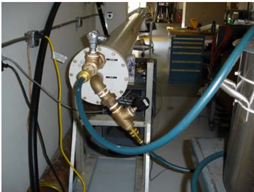
RF Load Water Inlet and Outlets
