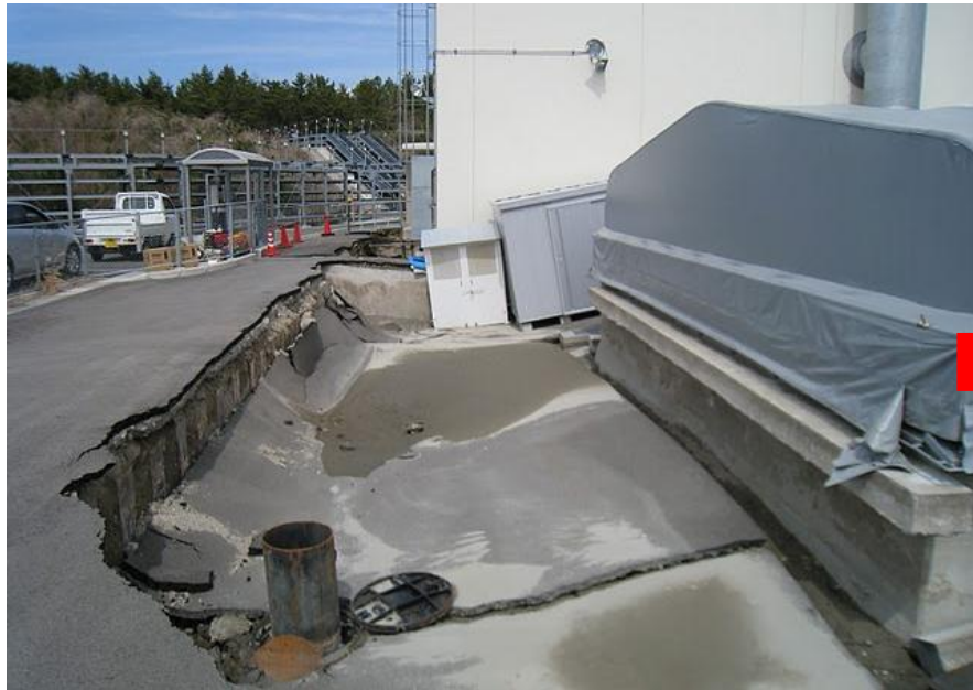
After Earthquake (Mar. 24 th )
