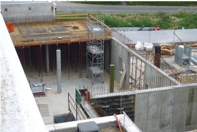
B199 (Cold Box) and B198 (Compressors)
