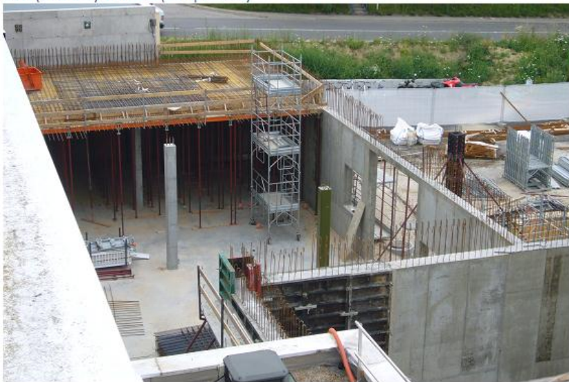
B199 (Cold Box) and B198 (Compressors)
