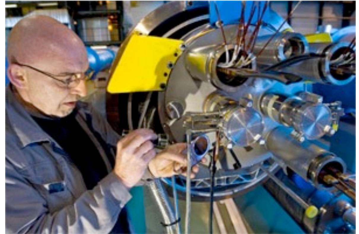
Final preparations on a replacement magnet ready to be lowered into sector 3-4
