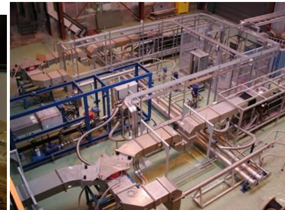
RF distribution: 2 MW CW 352 MHz
