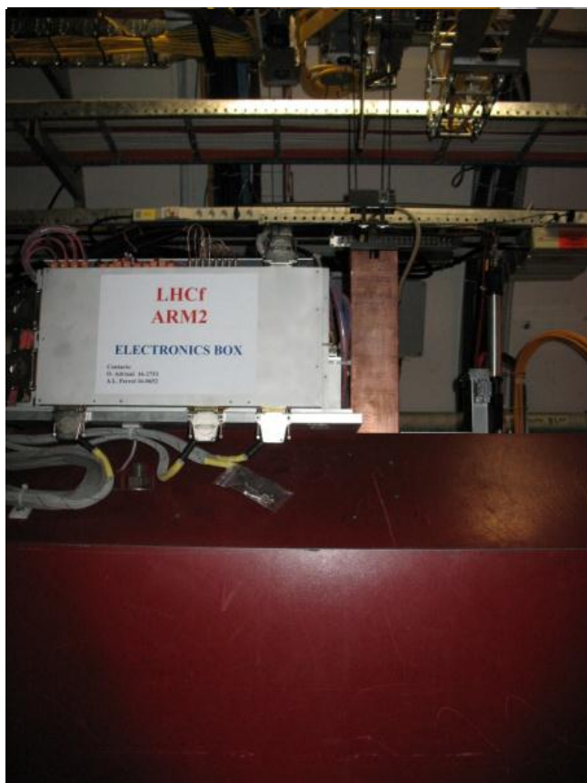
Point 1 remote handling system Installed in March 2009
