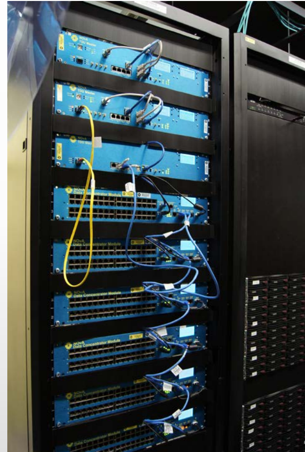
Master TDUs and test stand located in control room.
