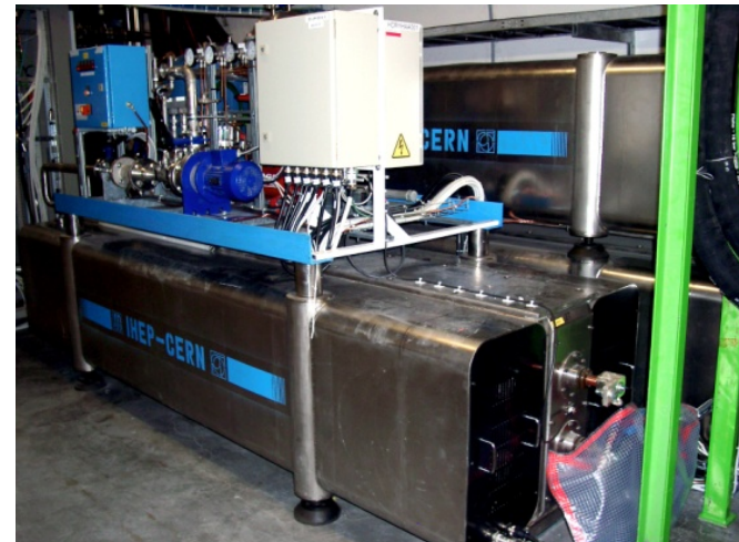
IHEP+CERN: Dump-resistors (77 units) - upgrade to accommodate twice more energy
