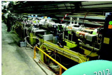
UA9 installation in the SPS
