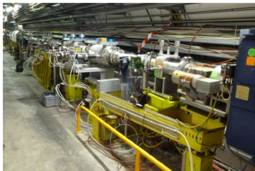
UA9 installation in the SPS
