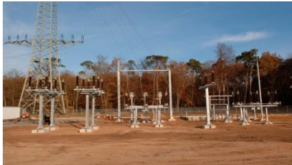
Power grid connection
