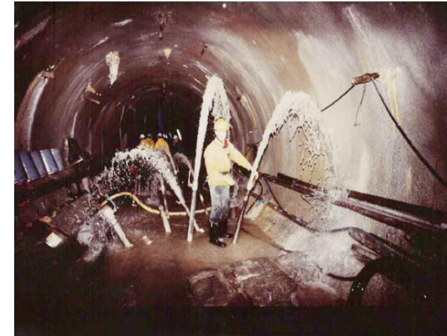
LEP tunnel collapse
