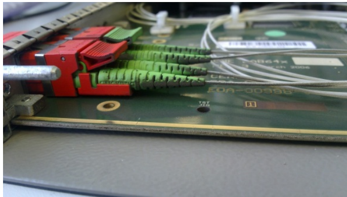
Accumulation of dust on the connectors
