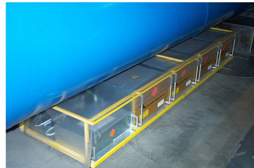
Figure 3: Protection rack type DYPB installed underneath the main dipoles.
