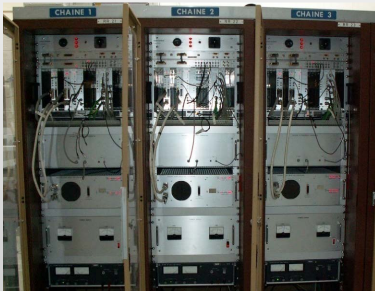
3 × peaking strip racks (powering & acquisition)
