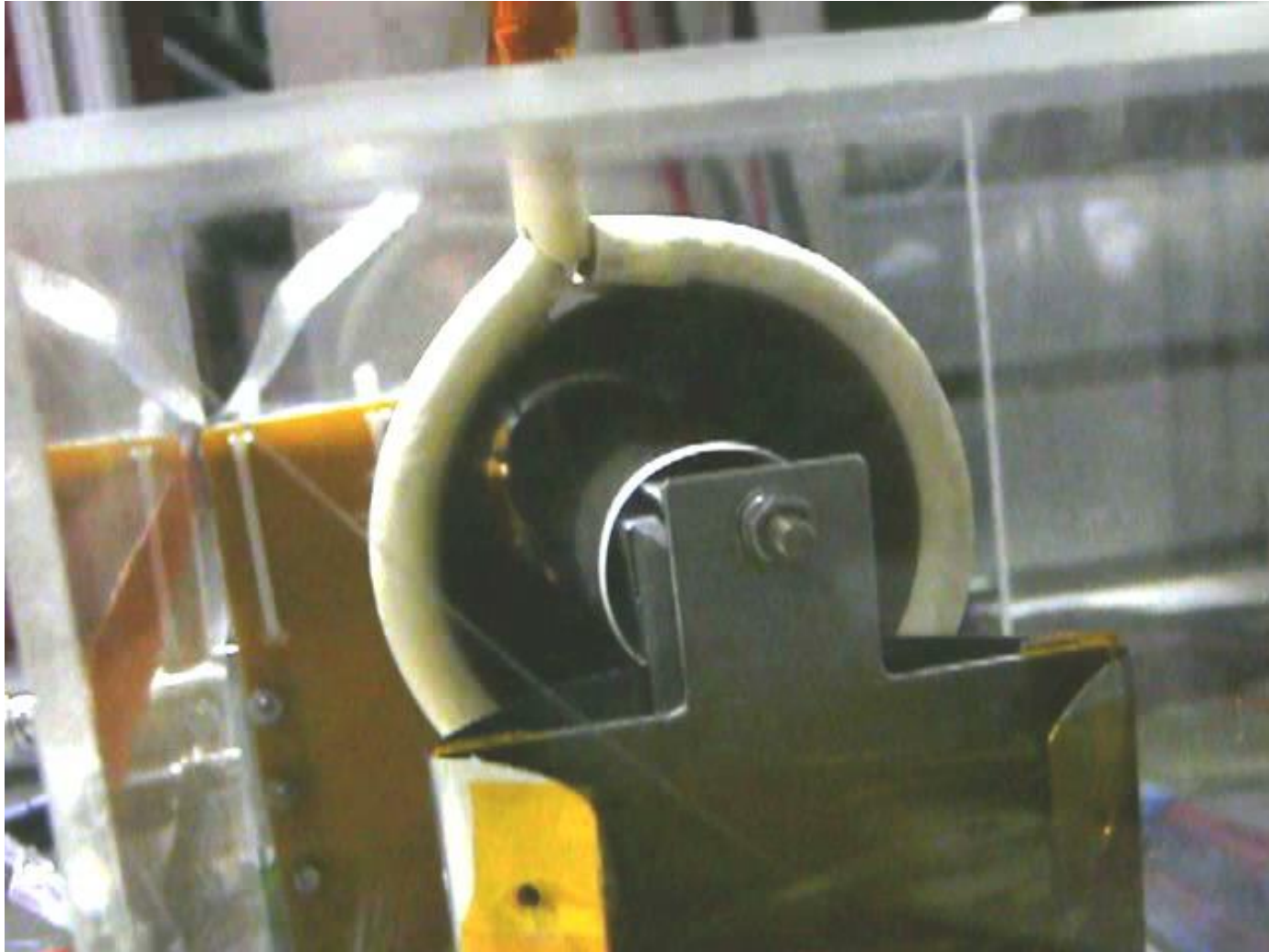
Arcing of HV Transformer
