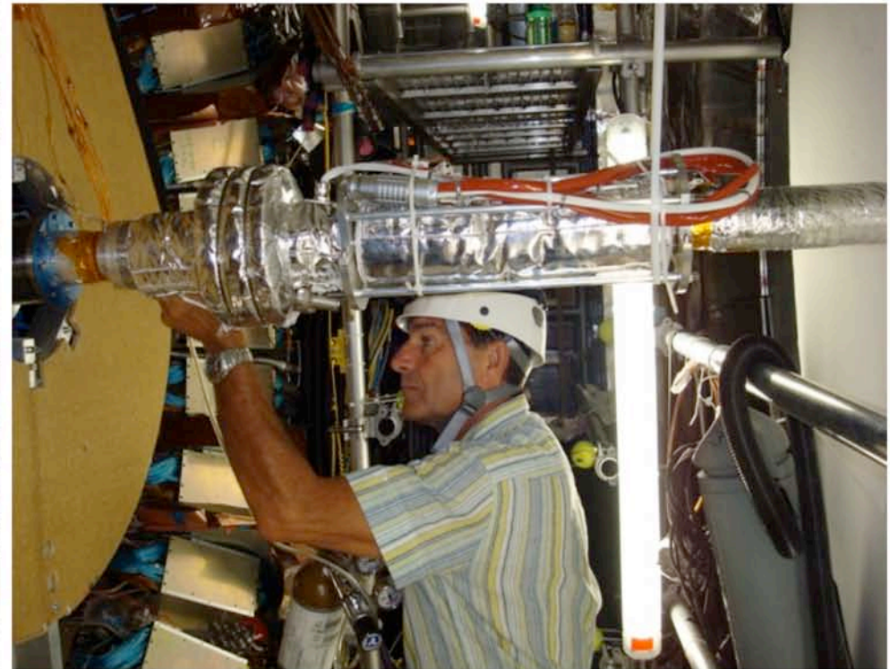
Connection of the ID section to the LAr EC beam pipe section
