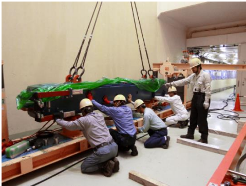
magnet installation for SuperKEKB;
