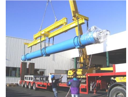
Unloading a 27 tons dipole
