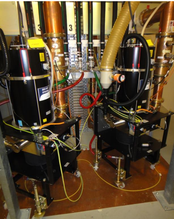
IOT installation at Diamond Lights Source
