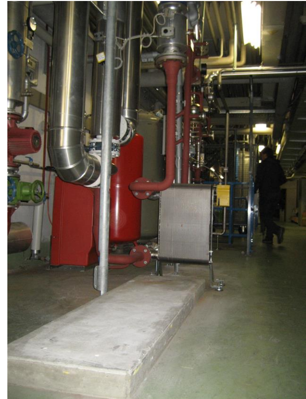
Existing heat exchanger with dT_m=5K (plate type fusion bonded, stainless steel) →very compact
