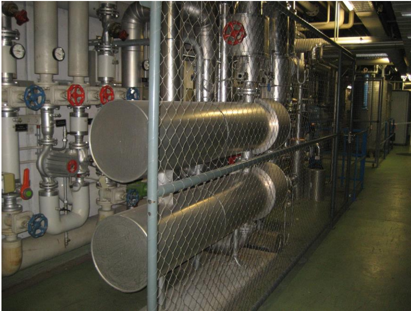
Existing heat exchanger with dT_m=22K (type pipe bundle)
