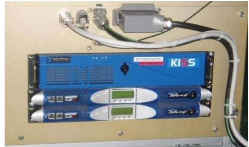
ACD FEC located inside HV generator
