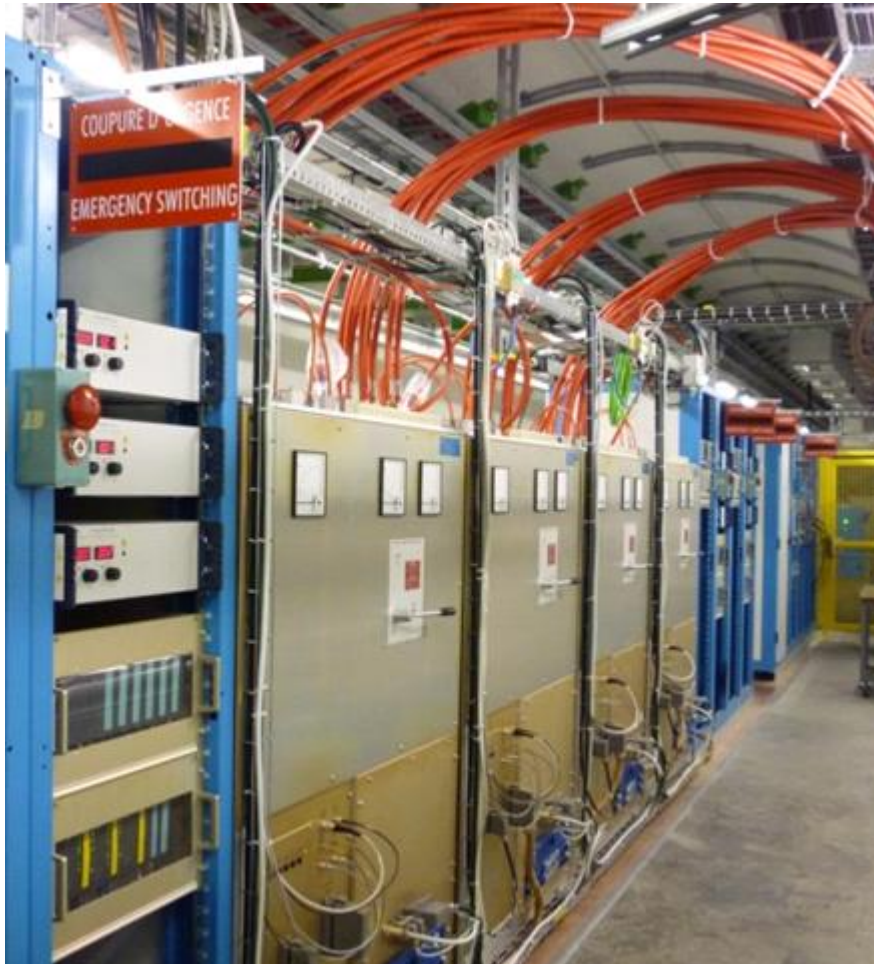
AC-Dipole installation at point 4 (UA43)
