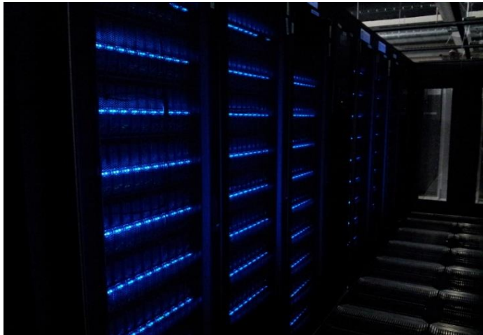
Panasas storage in RAL R89 server room
