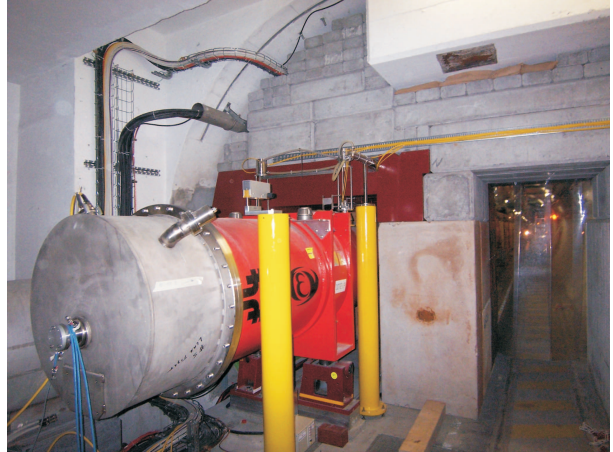
Figure 12: Machine background shielding in IR8, as installed at the IR1 side around the Q1 quadrupole (courtesy of D.Lacarrère).
