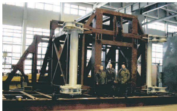
Figure 3: The frame of the blockhouse for the CMS forward shielding at the IHEP workshop (a photo from the IHEP Photo Gallery).
