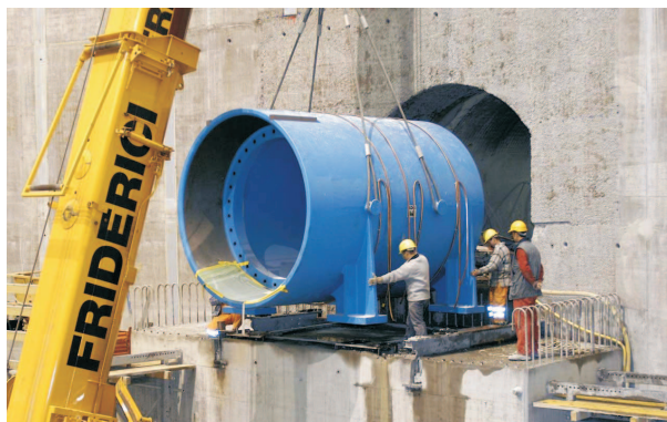
Figure 2: Installation of a part of the the ATLAS shielding in the UX15 cavern (a photo from the CERN Multimedia and Outreach Collection).
