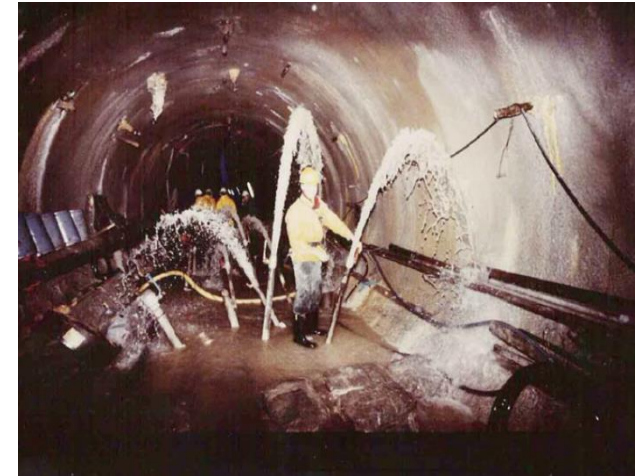
LEP tunnel collapse
