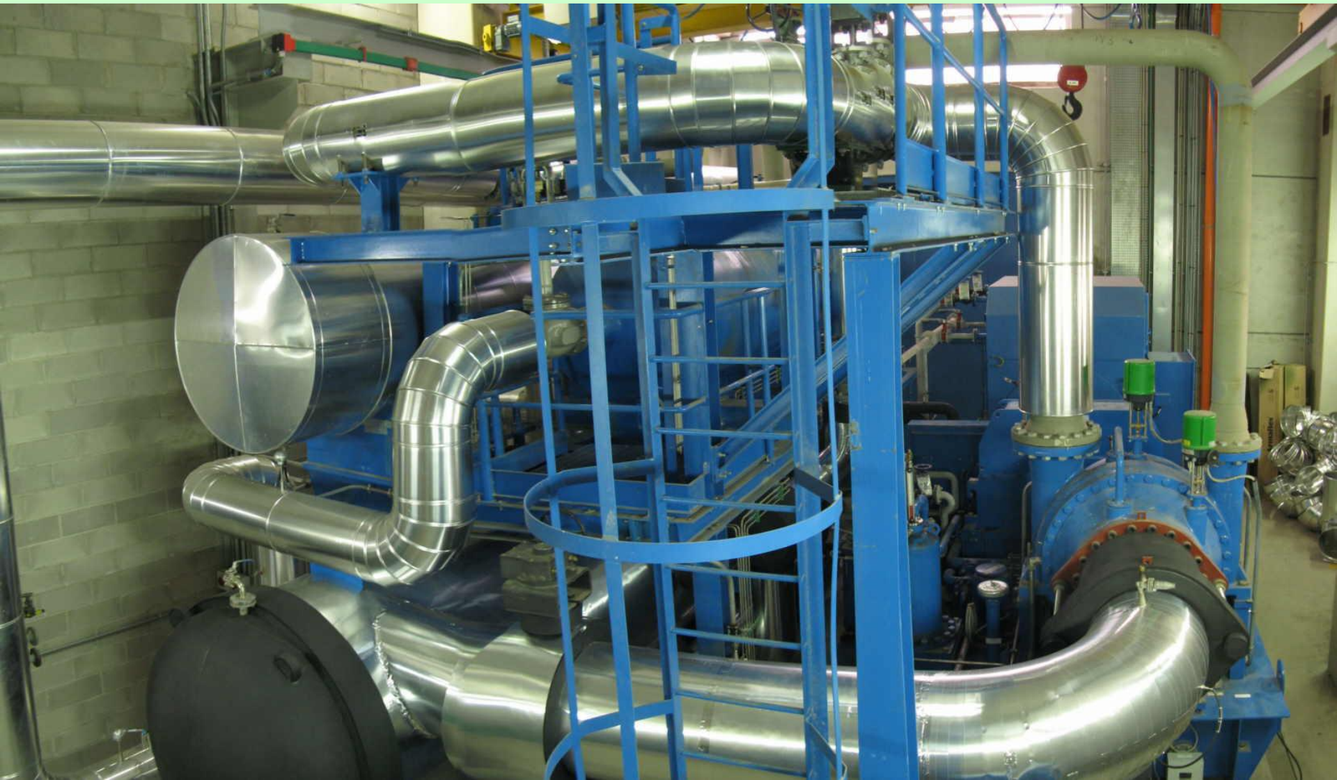
15 MW GROUND WATER HEAT PUMP WITH CENTRIFUGAL COMPRESSOR FOR A2A CANAVESE DISTRICT HEATING SYSTEM IN MILAN
