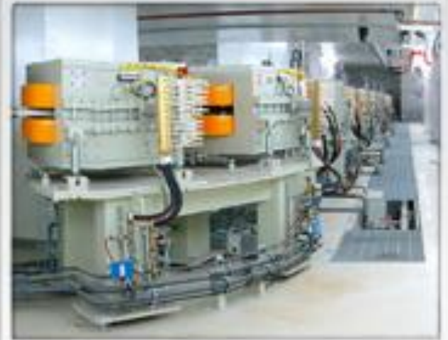
Beam Transport System
