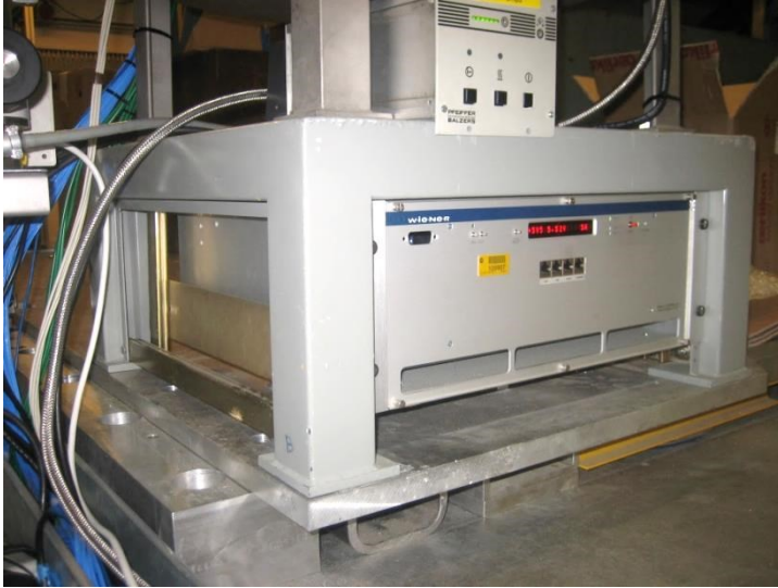
AFE PSU under cryostat
