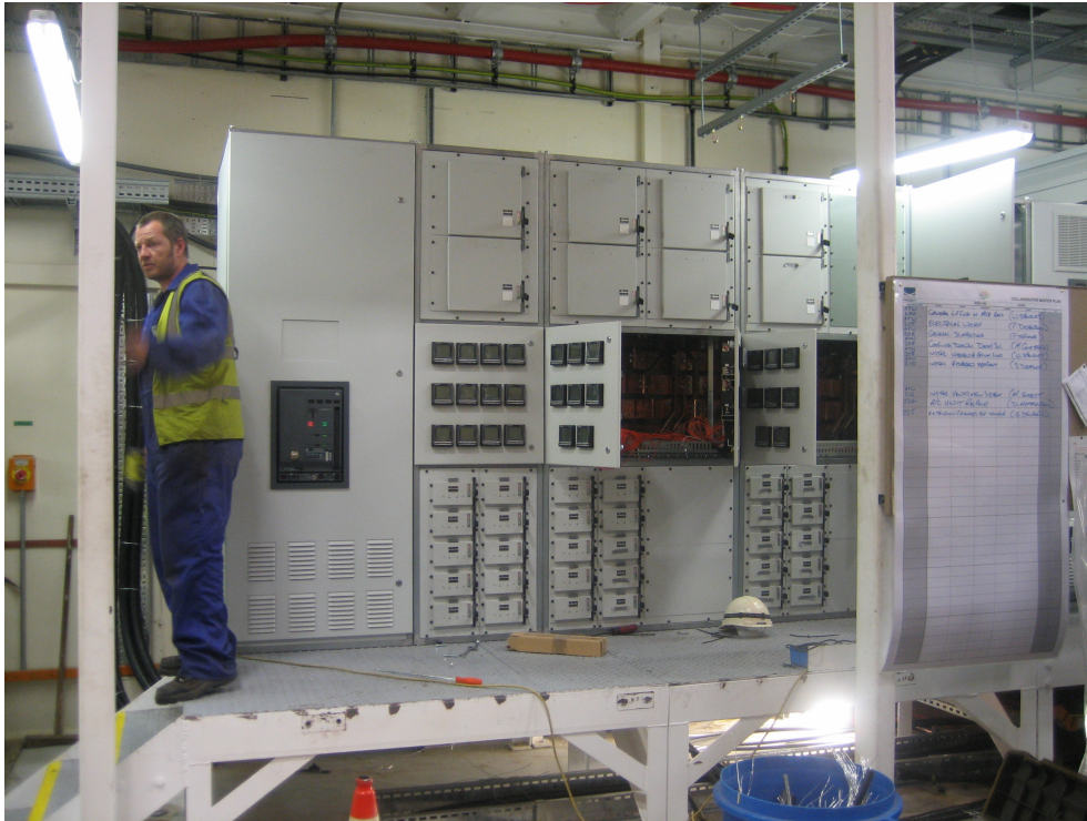
Figure 43: This photograph of part of the substation in the MICE hall clearly shows that a significant amount of electronics has been mounted in the front panels.
