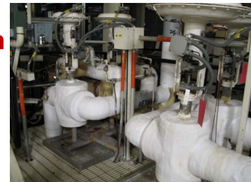
Control Valves on Inlet and Outlet of Each Zone
