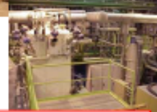
COOLING UNIT (CWU) and GHe HEATER Maximum cooling power is 120 kW. The warming up power is 200 kW.
