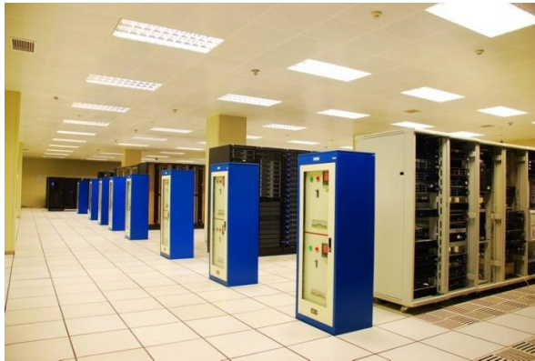
Power supply, cooling
