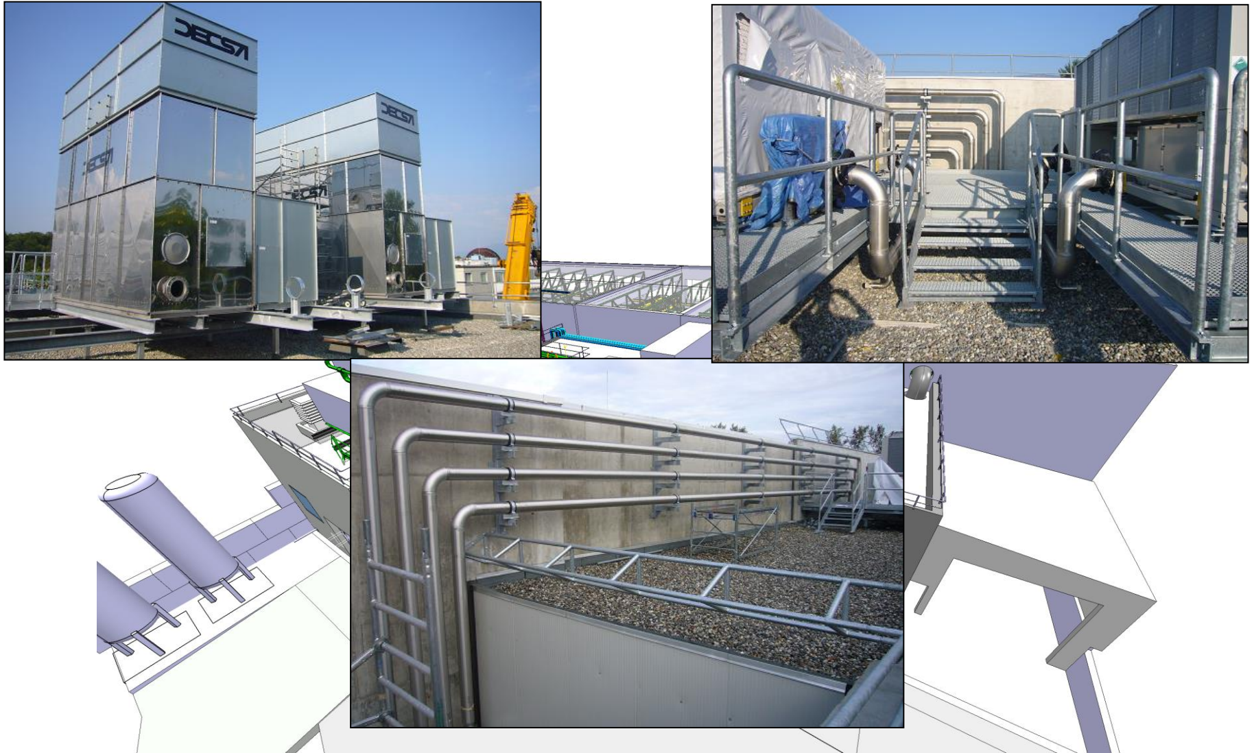
Cooling & ventilation: Cooling towers, Chillers and a large part of the tubing is in place 4
