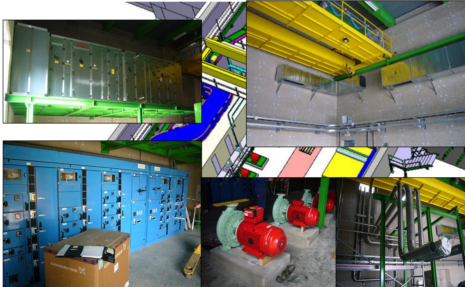
Cooling & ventilation and EL systems: Steel structures, Ventilation Unit, Electrical cabinets, Pumps and Piping in place as well as large parts of the ducts and cable trays
