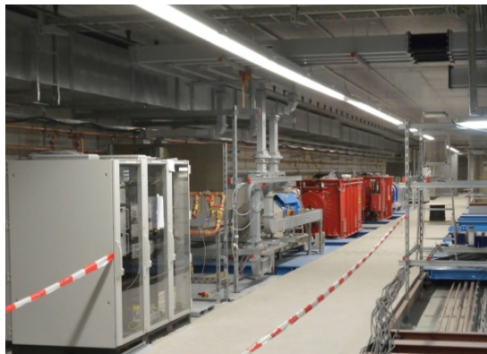
RF power components
