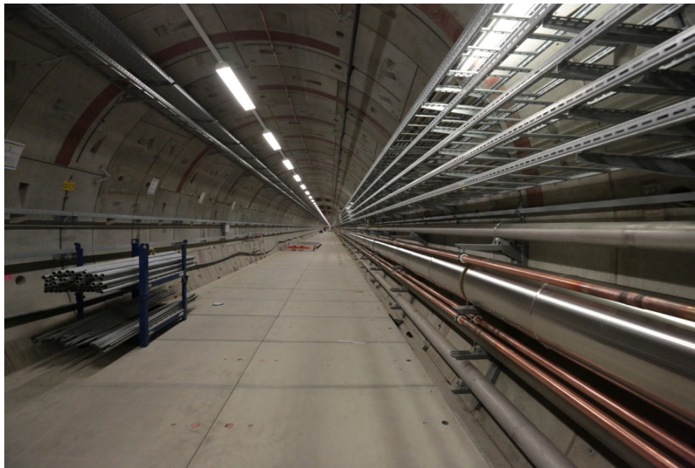
Utilities installed in accelerator tunnel
