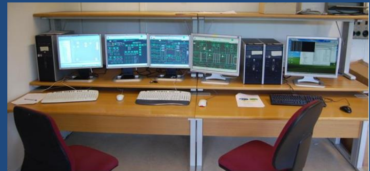
CERN CRYO Virtual Control Room
