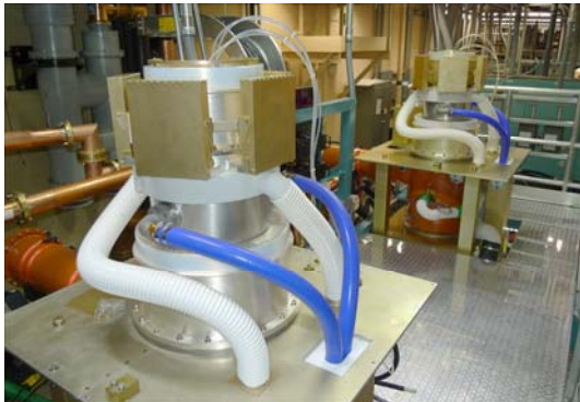
Figure 8. Two FPAs Installed, Diacodes in Center, Cooling Hoses for Water (Blue) and Air (White). Upper Blocking Capacitor/Slave Tuner on Top.
