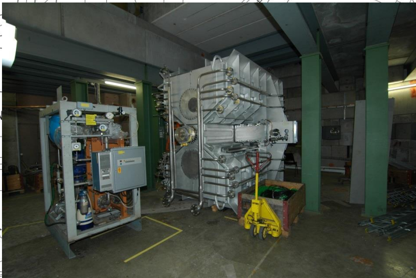
Resonator and cooling circuit moved to new test bunker
