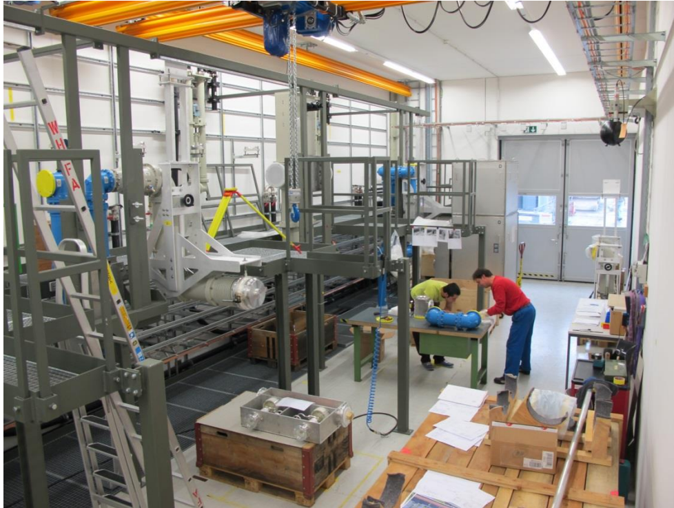
Installation in WHFA 9. Mai 2014
