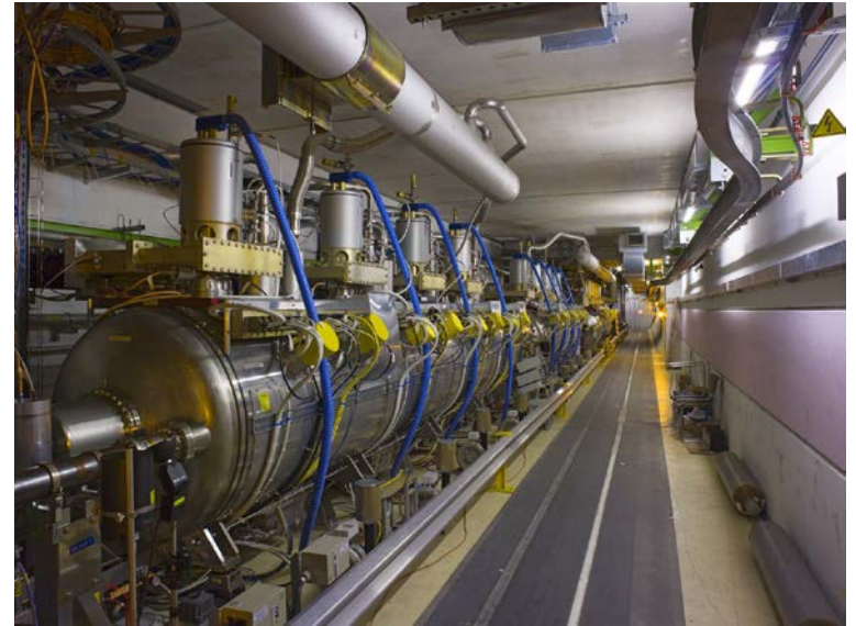
400 MHz Nb on Cu cavities in LHC tunnel
