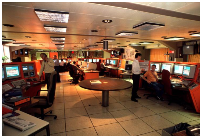
Control room of PS complex
