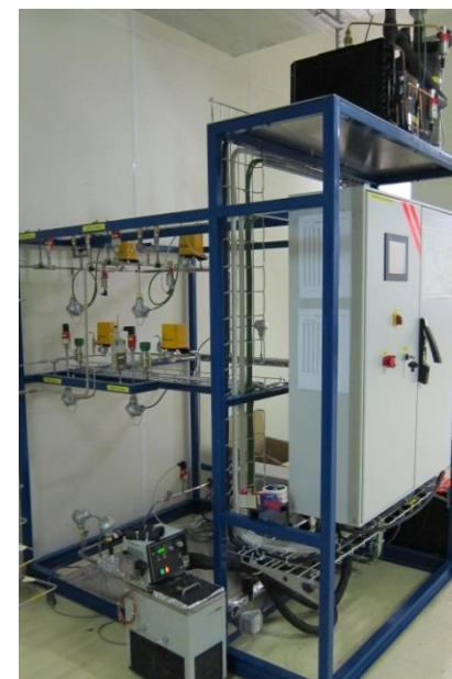
C 4 F 10 loop and plant.
