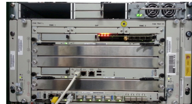
ATCA shelf to be installed in USA15
