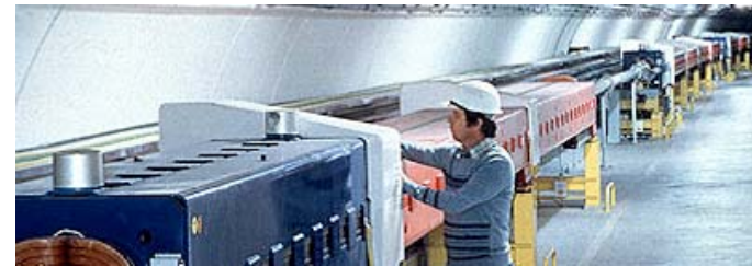
SPS was commissioned in 1976
