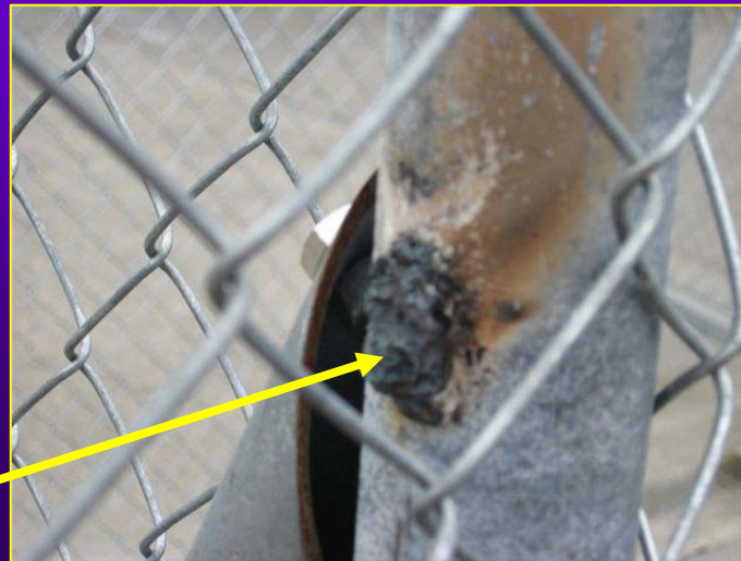
Melted bolt M10
