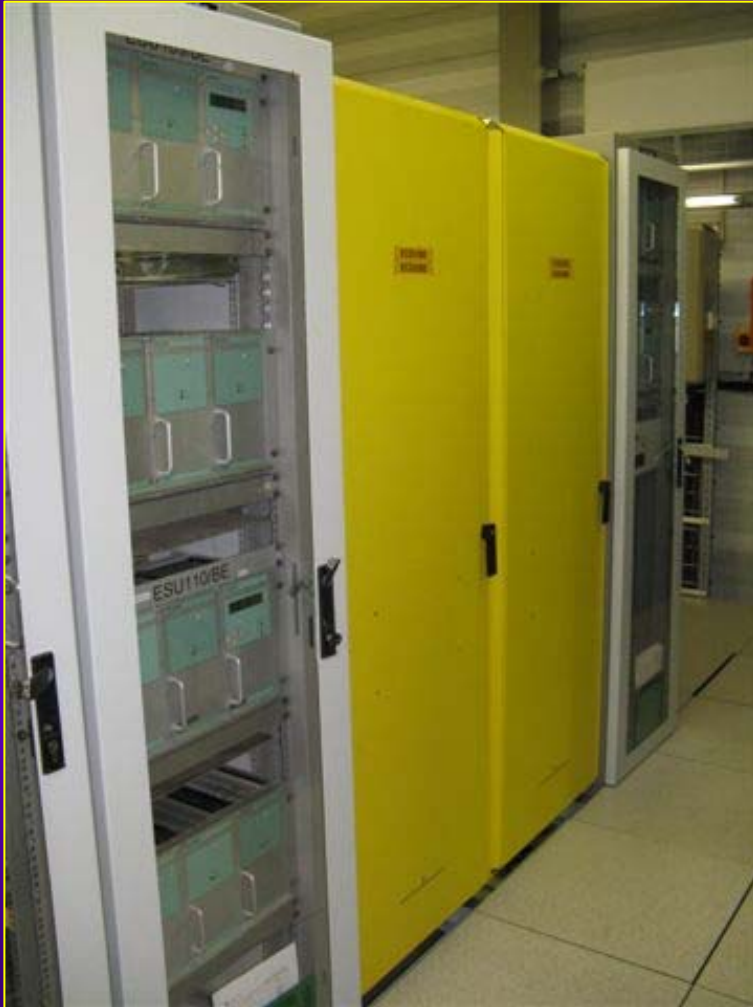
Auxiliary supply for 400kV station at CERN: Two redundant systems with automatic coupling
