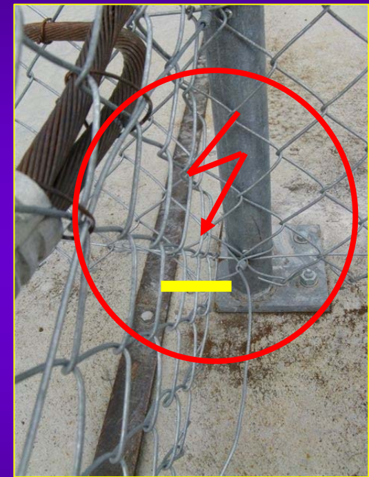
Cause: unwanted interconnection of two earthing circuits
