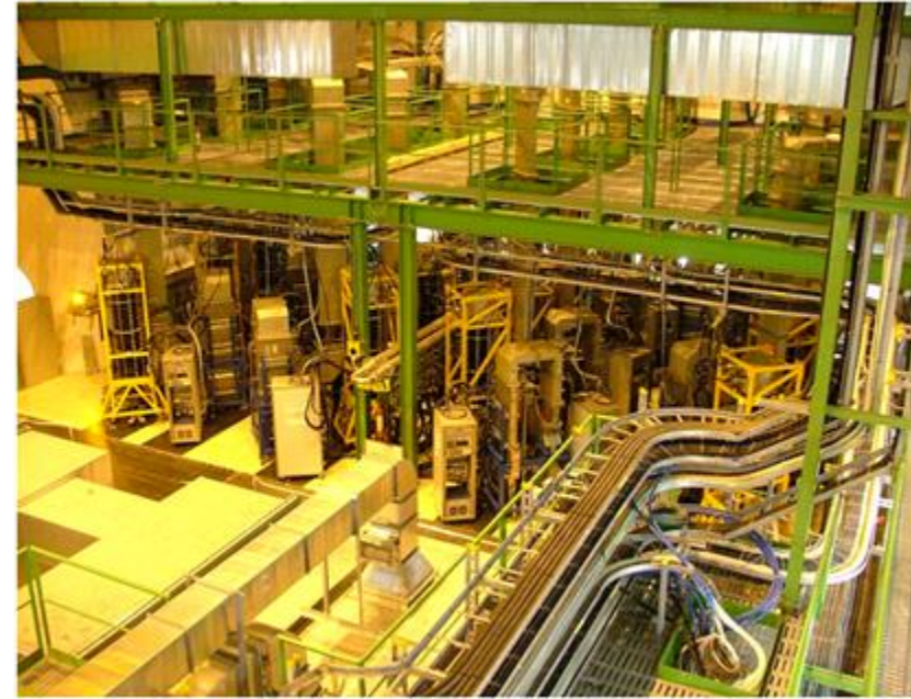
LHC 400MHz Klystron Installation
