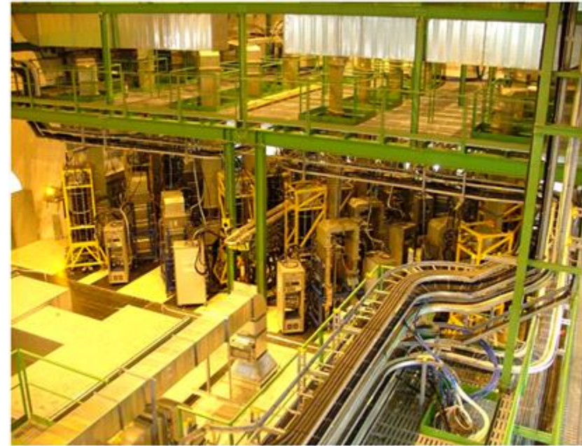
LHC 400MHz Klystron Installation
