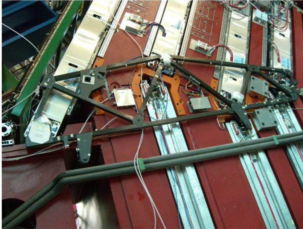
Close-up view of one of the platforms equipped with sensors and electronics
